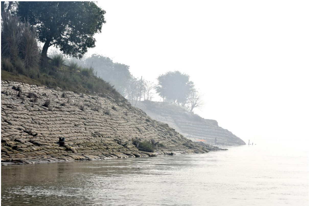
Image 33 : Use of Sandbags for controlling bank erosion near Patthar Ghat in Samastipur Distt.
